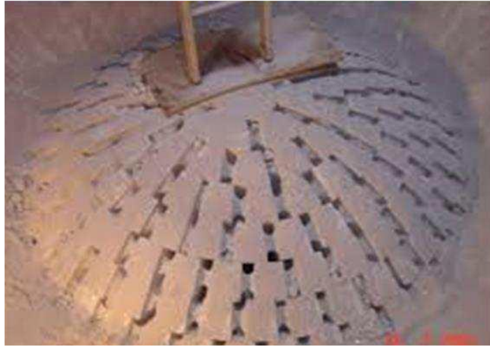
Figure 45 Hot Spots Due to Degradation of Refractory
