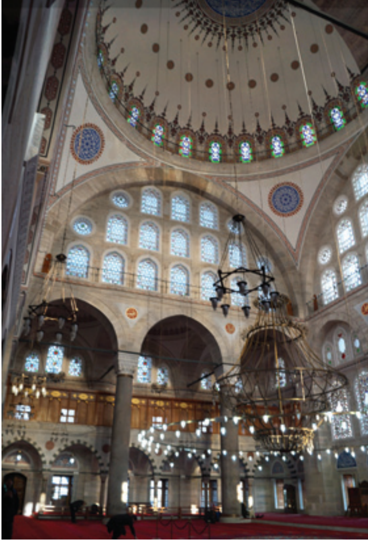
Fig. 3. Edirnekapı Mihrimah Sultan Mosque. The side gallery (mahfil) behind the main structural arch (photo: author)
