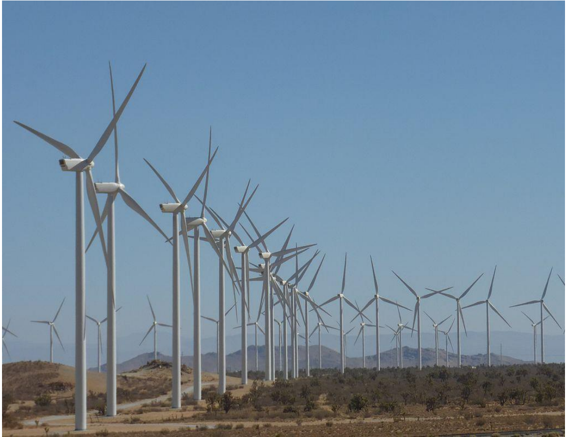
Figure 6: Gansu Wind Farm, China
